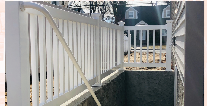
PVC RAILING WITH SECONDARY HANDRAIL
